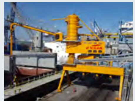
VIGAN NIV 600TPH/500KW INSTALLED AT THE NEW TERMINAL OF MASS CÉRÉALES AL MAGHREB IN THE PORT OF CASABLANCA.
