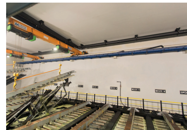
Figure: Energy chain for an indoor crane in a galvanising plant (igus®)
