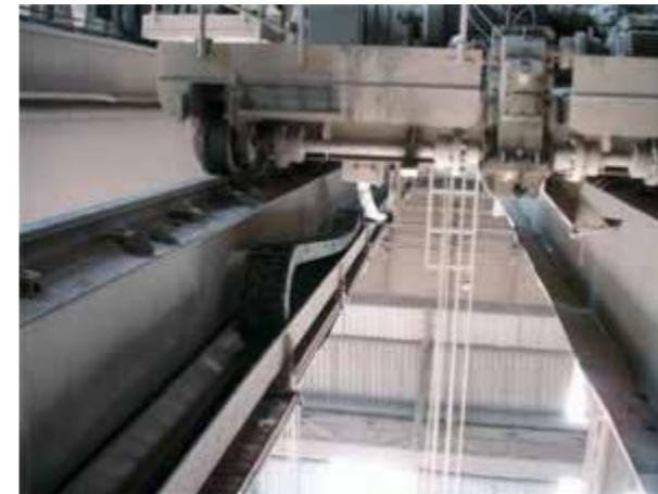
The same two-girder crane as above but after it has been modernised with a plastic energy chain in an aluminium guide trough. (Source: igus® GmbH).
