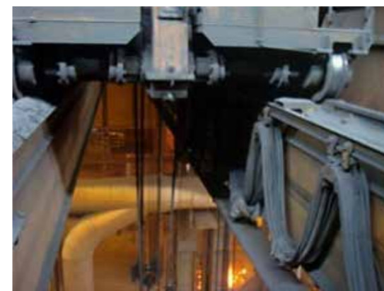
Energy supply via open hanging festoons on a two-girder crane. (Source: igus® GmbH).
